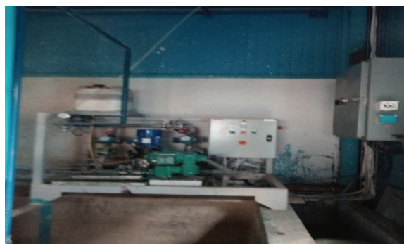
(b) Installation for polymer preparation
