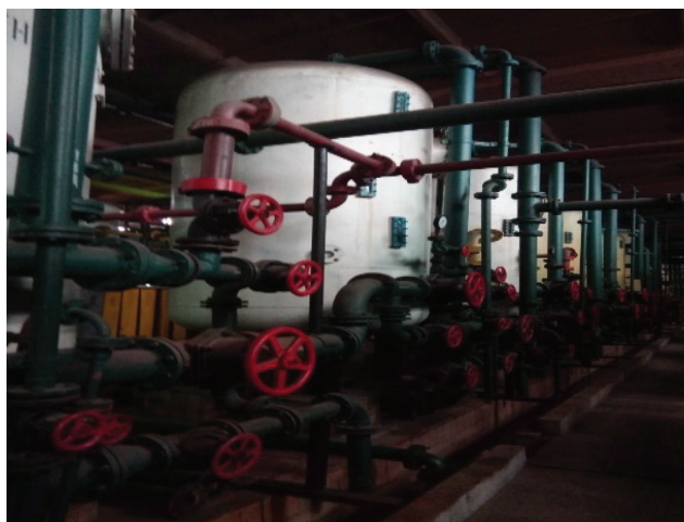
Fig. 3. View with ion-exchange filters
