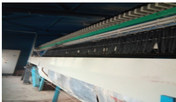
(c) Conveyor belt for sludge dehydration
